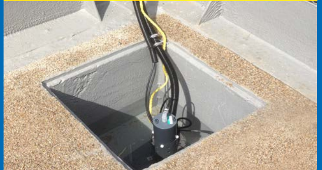
Sump Pump for Floor Voids under Timber Floors
